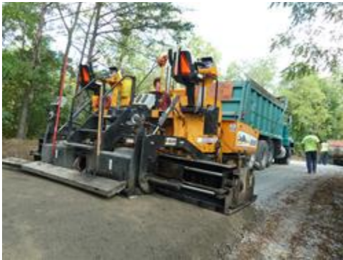
Left: Placement of Driving Surface Aggregate (DSA) with a paver from Mid State Paving during the Shale Pit Road rehabilitation project in Spring Township.
