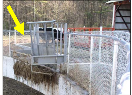
A farmer can utilize a manure storage stacking area connected to an improved barnyard. This beef farmer has a manure storage stacking area with 4 ft. concrete walls and floor (left).
