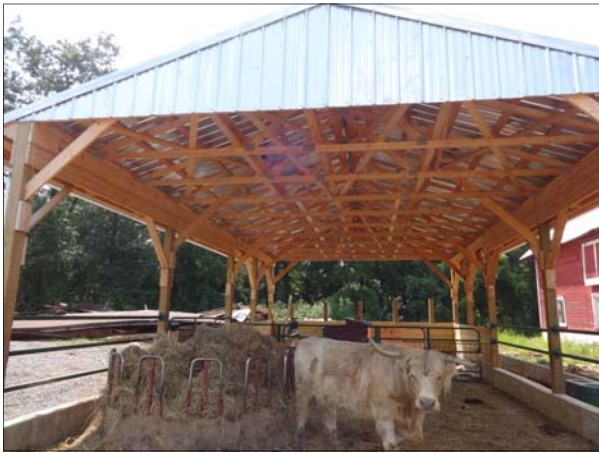
Two stand alone roofed barnyards/ACAs structures (above) and one barnyard/ACA with a roof extended from the main barn (below).
