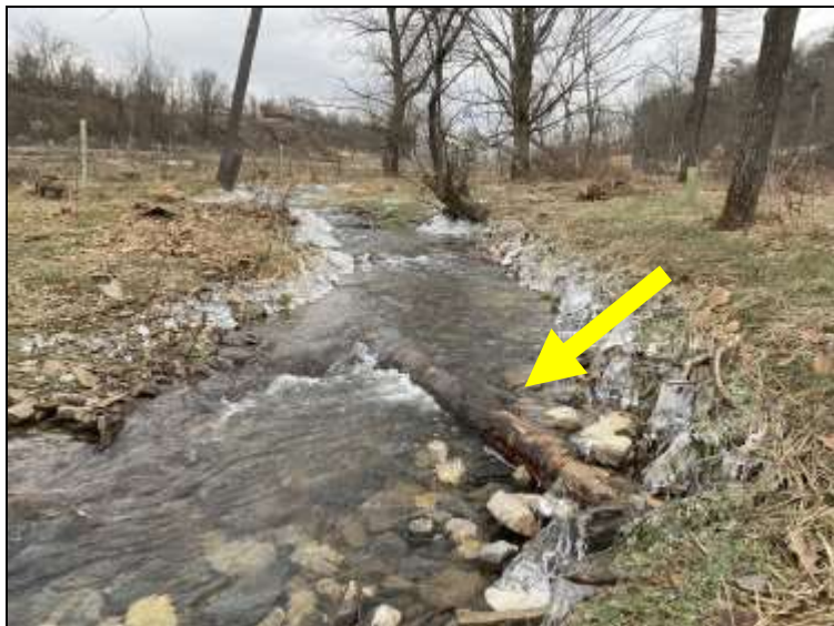
Single log deflector (top left photo, yellow arrow) installed within a stream.
