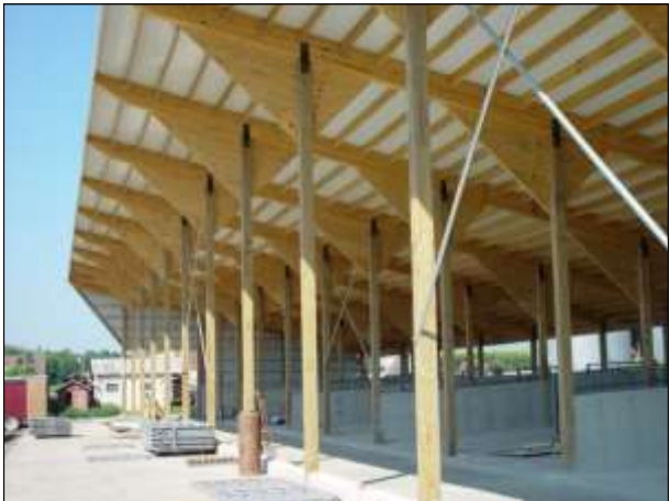
Although not funded by any public financial assistance grants, this farmer installed netting and a type of monoslope roof that prevents starlings from roosting in his roofed ACA (left and above).
