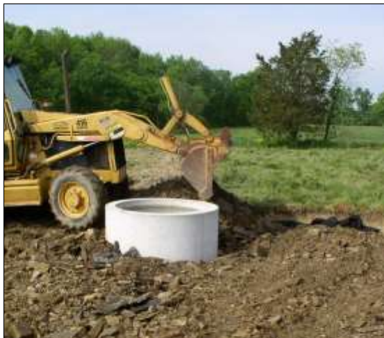
Base layer of stone being placed overtop of geotextile fabric around a precast concrete spring development trough on a dairy farm (bottom left).
