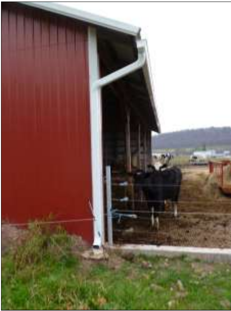
Underground outlets carrying roof runoff water can that outlet its water into a rock lined basin (mid-center) or lined with rock in some manner that is does not cause scouring (center left).
