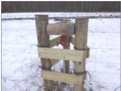
A frost free hydrant located in a pasture (bottom right). The bottom left photos shows a quick disconnect for a water line where water trough portability is preferred.
