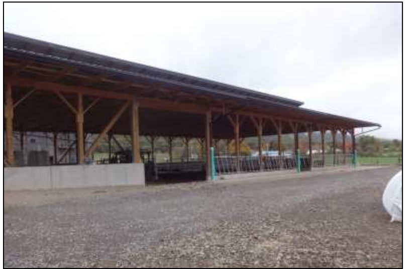
Example of roofs gutters and downspouts installed on a roofed ACA next to an improved barnyard ACA with concrete cubing (top left) and a roofed ACA on a separate operation (top right). Notice the green plastic pipe that will carry the roof water from the roof gutters and metal downspouts and transport it away to pipes underground.
